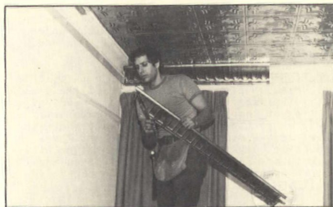
9. To make a neatly mitred corner, second piece of moulding is trimmed with tinsnips. Start cornice installation at corner furthest from door.
