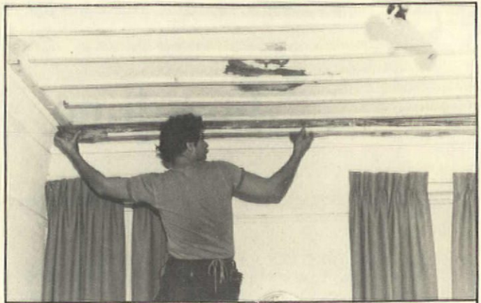
3. Additional furring strips are added, so that end result is strips that are 12 in. on centers. Strips are shimmed as needed to level the ceiling.
