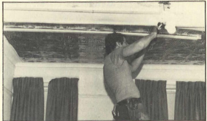
4. Metal panels are nailed to strips with 1-in. common nails, placing nails in the preformed bead. Mike holds loose end of panel with strip braced by his head.
