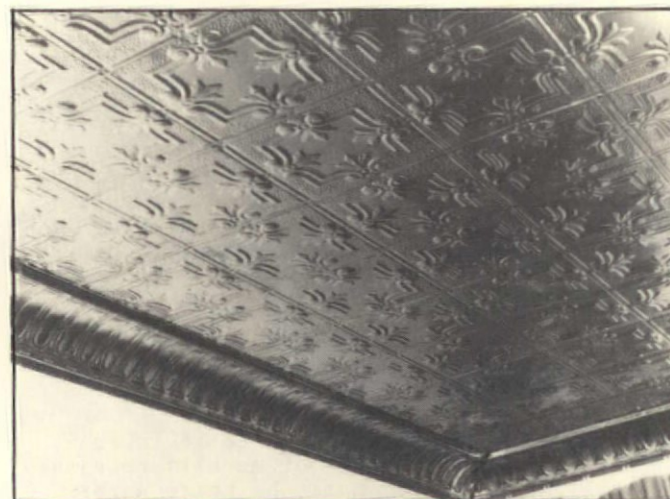
10. Any open seams are flattened by tapping gently with a hammer and a wide chisel or the back of a nail head. Caulk might also be needed for perfect closure.
