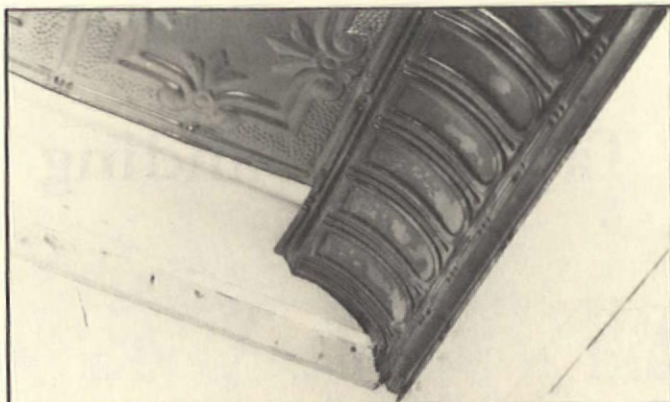
8. Metal cornice overlaps the edge of the last metal ceiling panel. It is nailed to the furring strips top and bottom with nails spaced about every 12 in.
