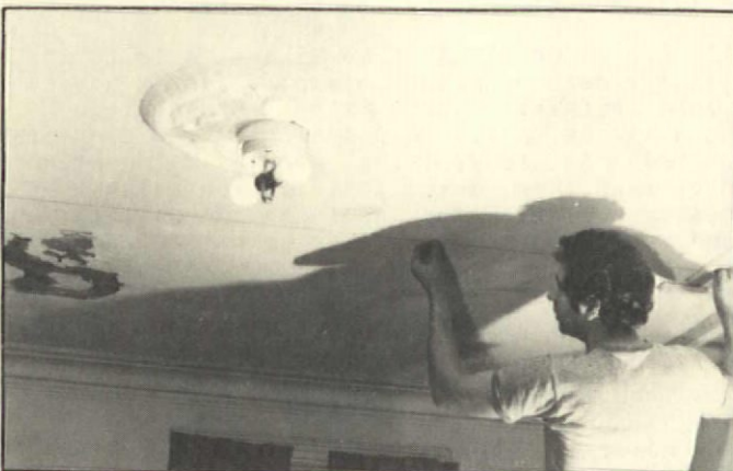
2. Furring strips are nailed around perimeter of room. Center of room is then located, and lines are snapped for the furring strips on 24-in. centers. These have to be located quite precisely because the metal sheets are rigid and can't be adapted to non-parallel nailing strips.
