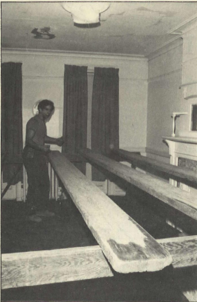
1. Mike Beck of C. A. Ohman, Inc., provides a steady work surface for himself by making scaffolding out of heavy planks.
