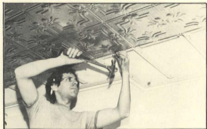
5. To secure ends of the metal panels, additional pieces of furring strip have to be nailed perpendicular to the long furring strips. This provides a secure nailing surface so that ends of the panels will lay flat.
