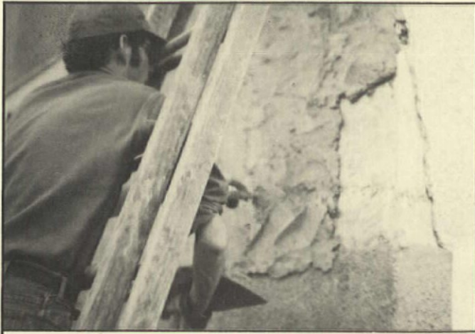
Don Minnery is applying the finish coat over the scratch coat. Dark section at bottom is the finish coat that has already been wire-brushed for texture. Light area to the right is the original painted stucco.
