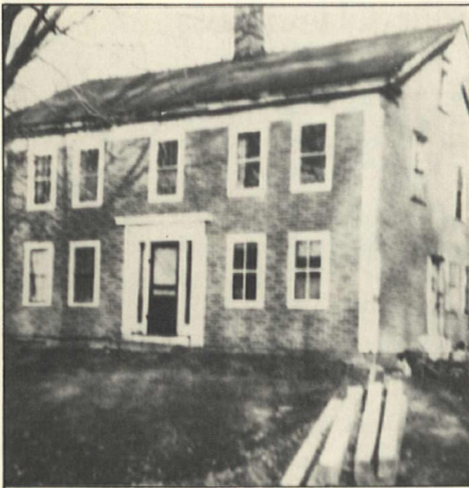
This is a snapshot of the Freeman house before roof restoration began.
