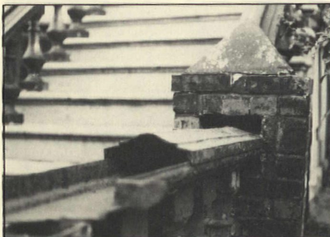
MASONRY REPLACEMENTS: Trouble begins when there's any fitting of cast iron parts into masonry. Masonry absorbs water, causing metal to rust. And the interface between the two unlike materials creates a visual problem, especially evident in the bottom photo. Simple butting of masonry against iron is not so troublesome. Again, though, there can be a problem with the way it looks. In the top picture, the proportion and detail are fine, and the whole assembly is painted with brown sand paint to look like carved stone. The middle example lacks finesse.
