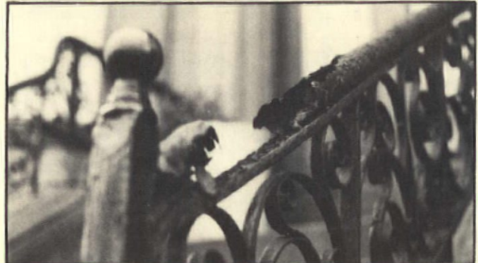
This kind of advanced corrosion prompted the ad-hoc replacement, below.
