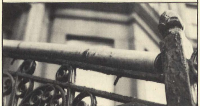
Note visual problem in connecting old to new. Pipe end could have been cut to fit.
