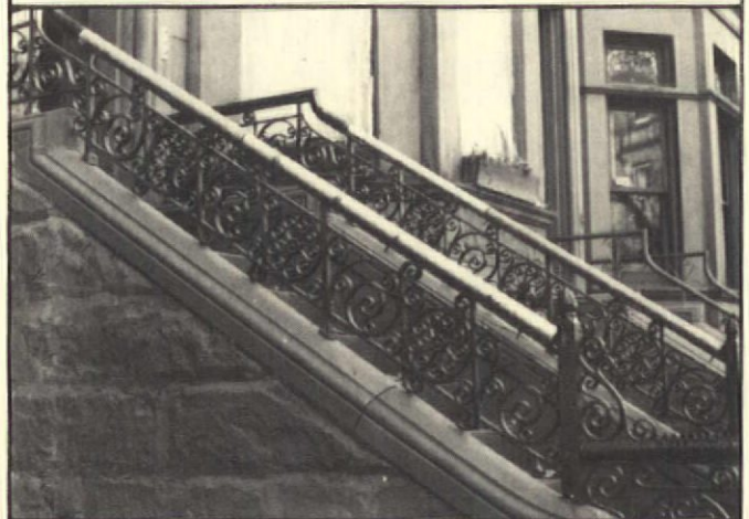
Simple replacement with galvanized steel pipe seems an ingenious and cheap solution.
