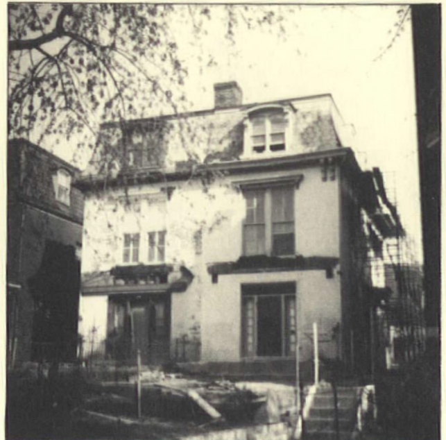
1978, and both the Giordano's porch and the porch on the attached house are off.
