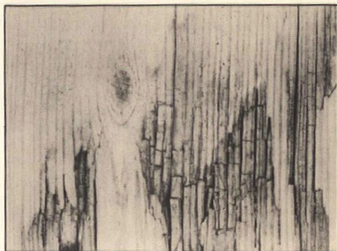
Brown rot occurs most often in softwood --and thus is the rot most often seen in exterior woodwork. Brown rot is characterized by cracks and checking across the grain.
