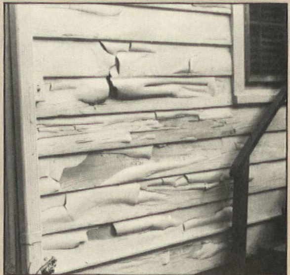
Peeling paint denotes major moisture problem, in this case from a clogged gutter. With wetting of this magnitude, rot will not be long in coming.
