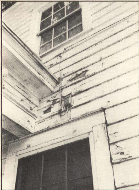
Peeling paint tells the story: Porch roof diverts water against the side of the house. Note decay starting where siding meets window trim.
