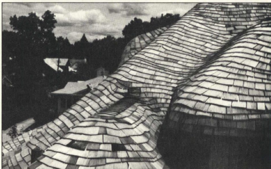
Views of a new wood-shingle thatch roof in Sioux Falls, South Dakota, laid by C & H Roofing. The original, unique roof structure, together with a rediscovered shingling method, create a roof that is the major architectural feature of the English cottage-style house. Can you imagine such a roof covered with any modern material?
