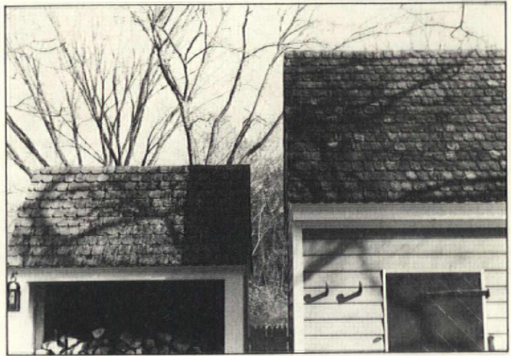
Two outbuildings in Colonial Williamsburg: One of these wood shingle roofs is an impostor. Can you tell which one is the real wood shingle roof? *
