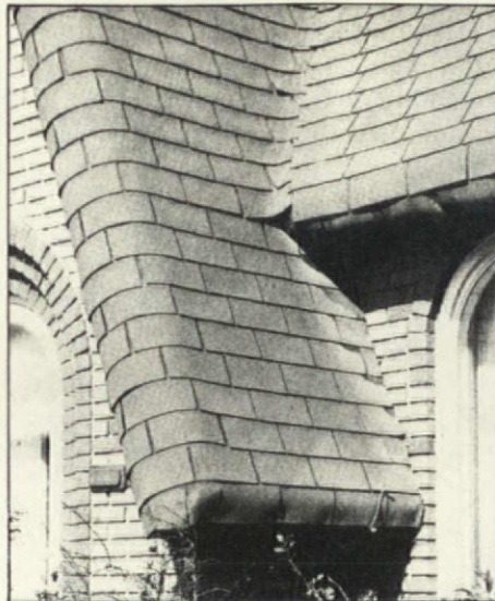
The sad but common condition of 'thatch' roofs today: Cheap, clumsily applied asphalt shingles never look worse than on these undulating roofs.
