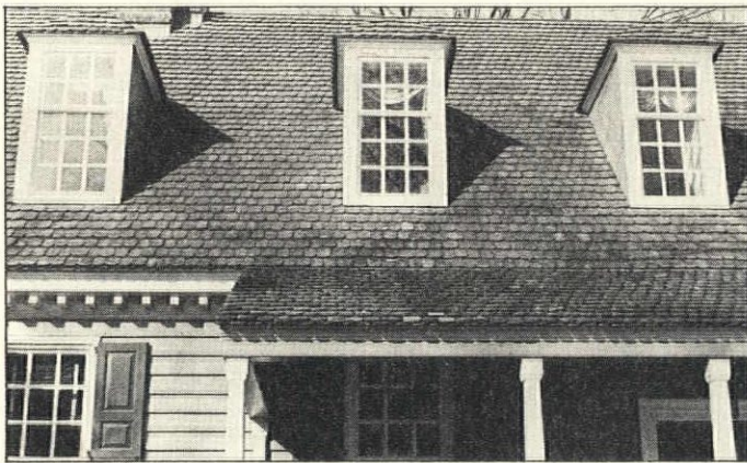
These asbestos-cement shingles would not arouse suspicion in the average visitor to Colonial Williamsburg.
