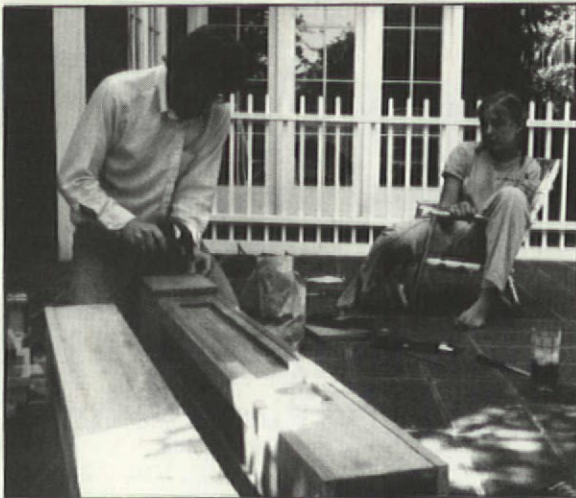
The author and daughter Wendy are shown attaching the base trim to a built-up post column using butt joints.
