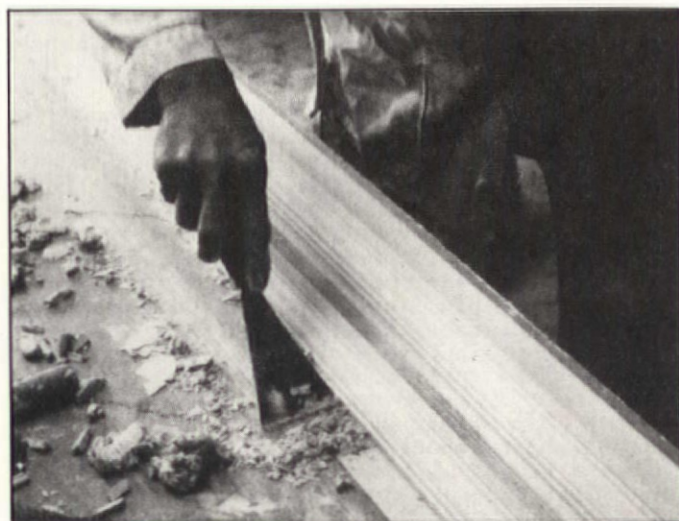
Step 8: Use a putty knife to scrape away thin plaster left on the surface of the bench after you've finished running the moulding.
