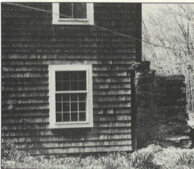
Stephen Sterling's 1786 addition to Sterling Heights was built on somewhat swampy land. Sometime early in the 19th century this stone buttress was erected to help support the house.
