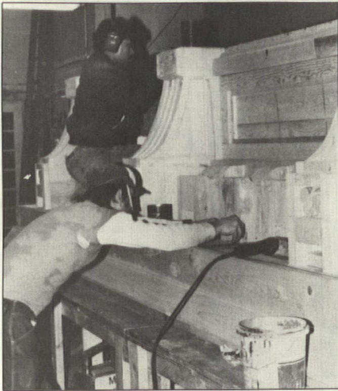
Two workmen are attaching decorative brackets and modillions to a cornice being built in Michael Pangia's shop.
