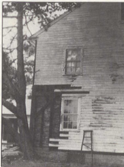
The exposed post was rotted and had to be repaired. Note the tripled 2x6s used to replace a rotted section of the sill.
