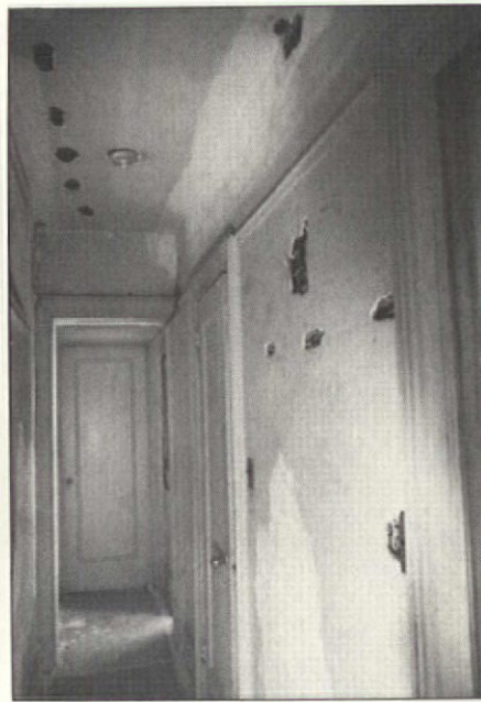
Here's graphic proof that you should never repair plaster until the electricians leave. Indirect light has already been installed.
