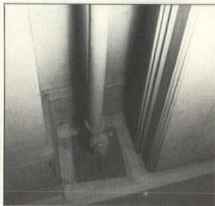
The naked riser before we added a fluorescent fixture and Sheetrock baffle.
