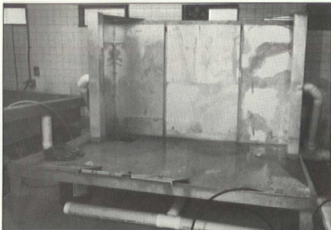
The water-rinse booth.
