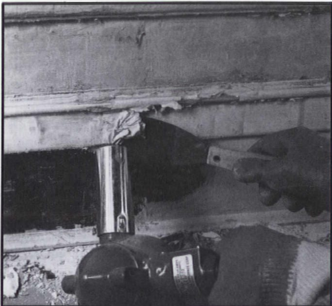
Here, a heat gun is used to melt multiple layers of paint off a baseboard.
