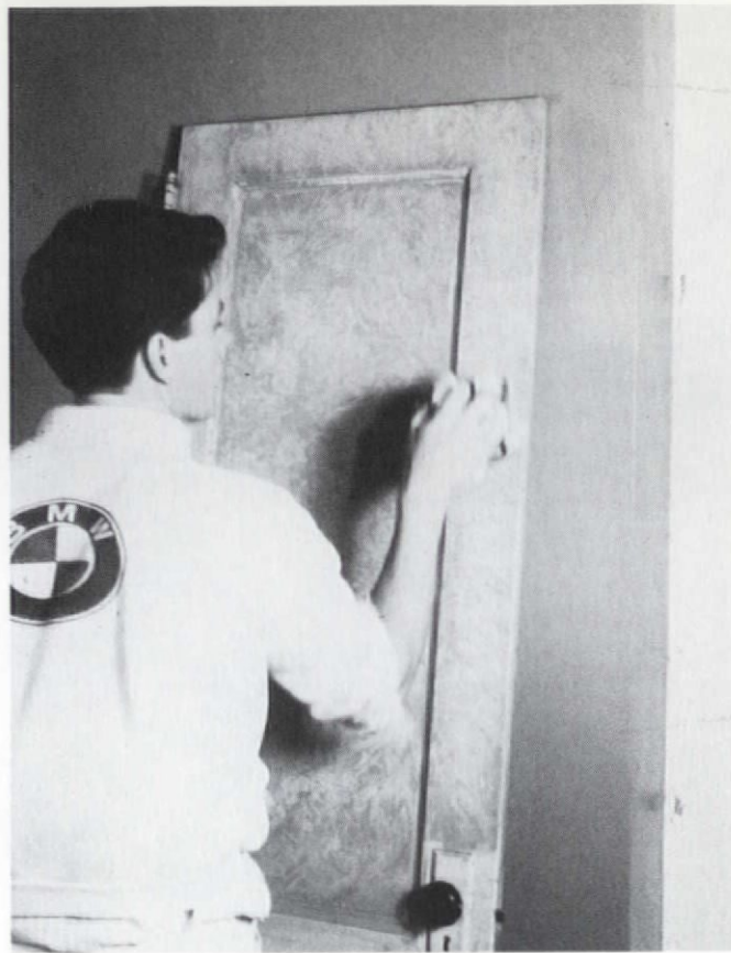
Here’s the rubbing technique used on a door. The center of the panel can be rubbed more than the panel moulding, giving subtly different densities of the same color.
