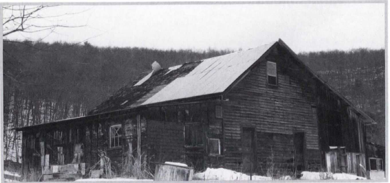
The entire building may need work, but stabilizing a leaky roof is the first critical step.
