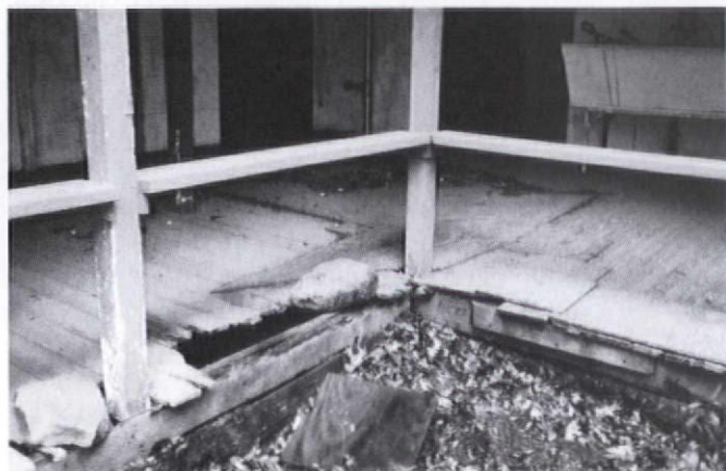
The back porch is now rotting away
