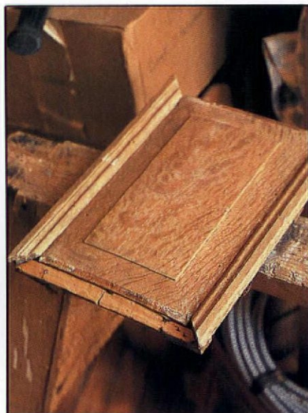
Applied panels were originally toenailed from the hidden side of the wainscot. Many were damaged by previous "restorers" prying them off.
