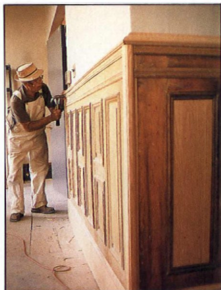
Missing panels: Cut on a table saw with an ordinary combination blade. After blade angle and depth were set, panel was run through on edge.
