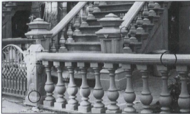
Well maintained cast iron: All repairs were done by owners as soon as problems appeared. Detail below.
