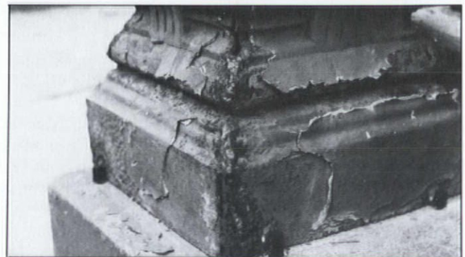
A professional repair job: The small tabs at the base of the newel are welded to the iron and set into holes in the masonry for stability. This is a shortcut job — the tabs should have been welded on the inside, where they'd be less conspicuous.
