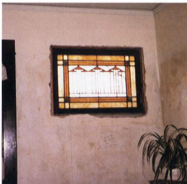
One of the walled-in windows, fully lit again after 50 years in the dark.
