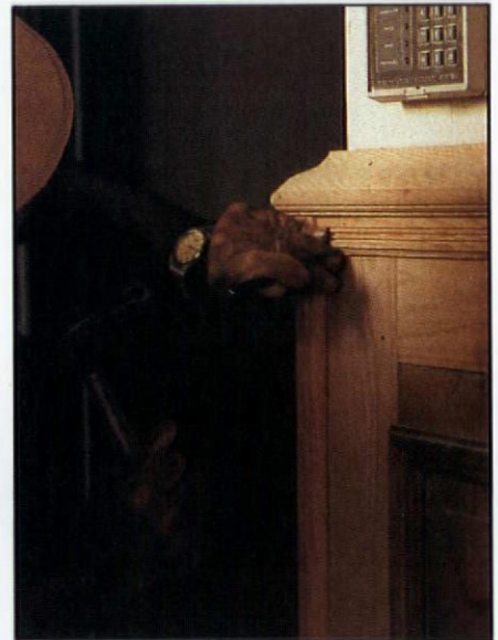
The 8'-long top rail was spliced; the corner guards (all missing) came from appropriate stock patterns in oak. Nail beads were set, then filled.
