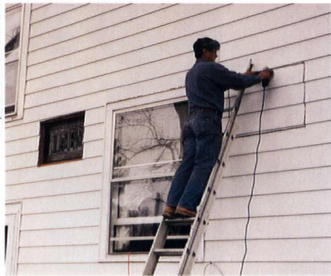
Careful work on inside and outside walls uncovered two c. 1917 art-glass windows.
