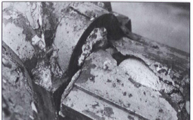
An example of exfoliated iron expanded by rust due to filling with concrete.
