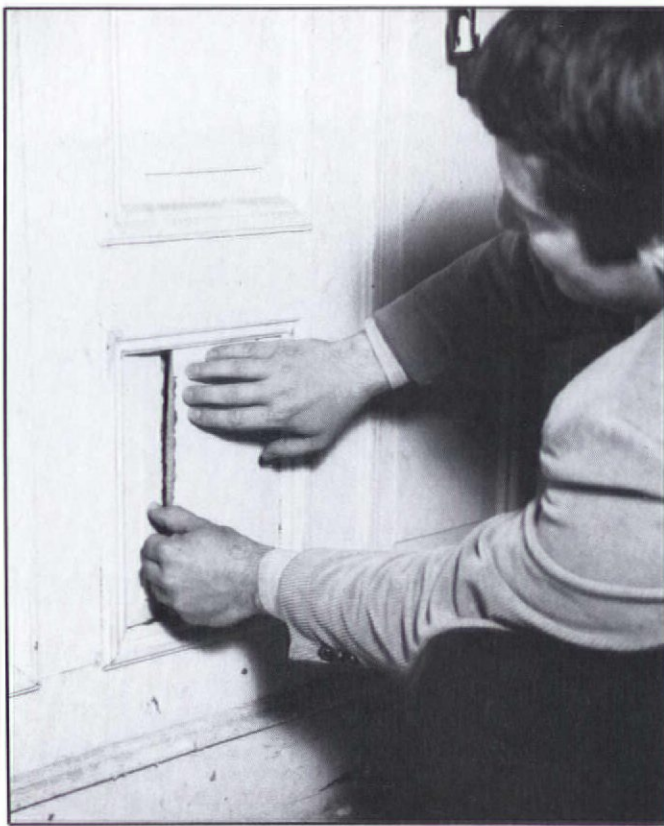
This panel had a hairline crack the owner may have been tempted to fill with paint. But a closer look showed it was completely unattached and ready to fall into the wall.
