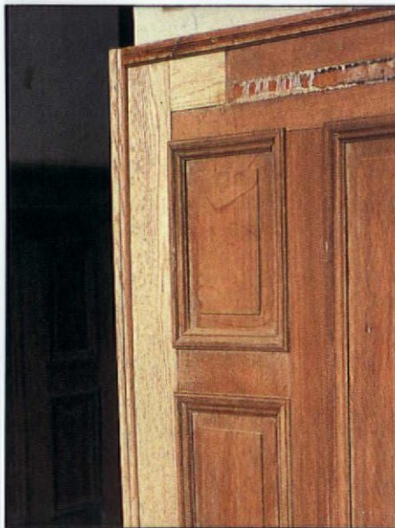
Alterations, wear, and the "missing-pieces syndrome." Trim expert Vito DiDonno began by rebuilding the (accessible) outside corner.
