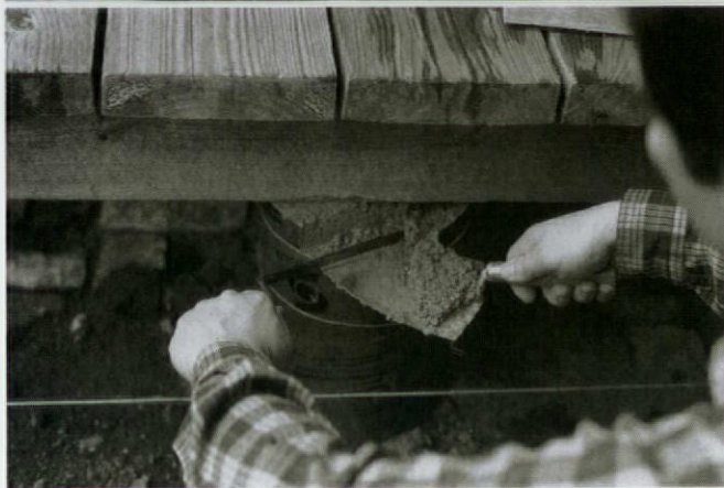
To fill a tube to capacity using a door, slide the door up the tube in stages as you add concrete mix (top), then top off the tube when the door is at its maximum height (above).
