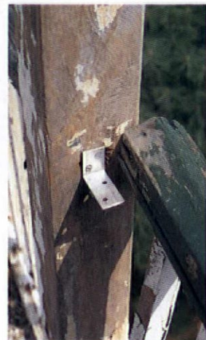
Knee plates mount to the porch support first. Then the rail (mortised at the end to accept the plate) is angled on and attached from below.
