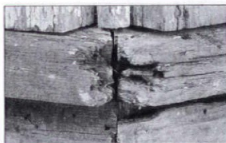
This rotted - and irreplaceable - woodwork...
