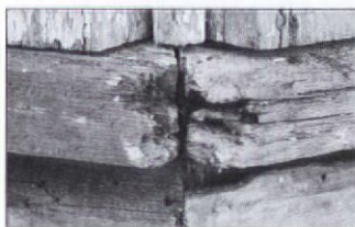
This rotted - and irreplaceable - woodwork...
