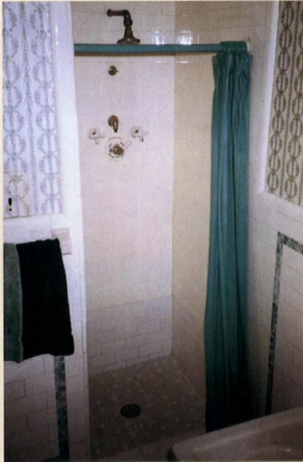
Above: a post-repair shot of our shower stall. Prior to the mud job, the subfloor had sunk a full 3/8" because rotted joists could no longer support it.
