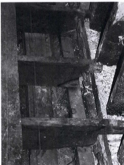
Weakened masonry and framing typical of the ailing substructure we found in areas around the building.
