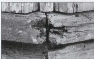
This rotted - and irreplaceable - woodwork...
