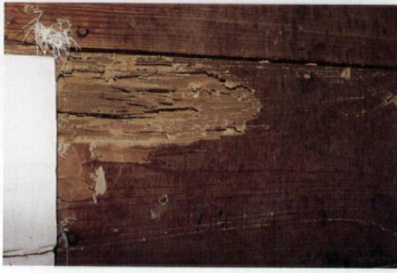
Top: These shelter tubes, built under siding and building felt, are evidence of an old subterranean termite infestation. Above: Characteristic subterranean-termite damage: extensive tunneling with the grain, which leaves much of the harder winterwood intact. Ordinarily, these insects would never have penetrated the wood surface, but this damage, high on a first-floor wall, was originally protected by wallpaper.
