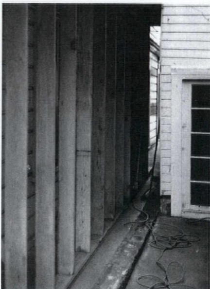
The completed shoring wall, viewed from the next lot. The foundation runs down the middle of the photo.
