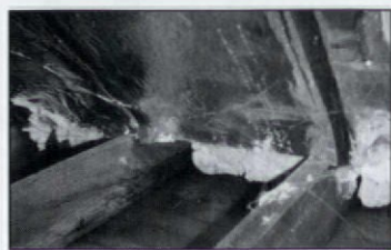
Urea-formaldehyde foam in an attic installation.
