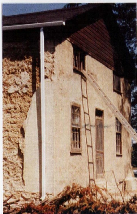
As mud eroded behind it, large chunks of 1950s substitute siding detached from the walls, revealing extensive exterior damage.
