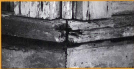
This rotted – and irreplaceable – woodwork...
