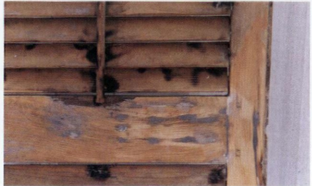
A prime coat of thinned resin consolidated the damaged wood and provided a strong surface for the filler to adhere to.
