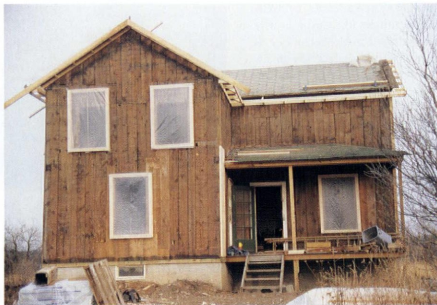
Siding off, the vertical planks supporting this house without corner posts become clear. Note the joist pockets near the windows.
