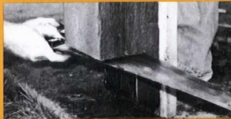
10" rotted bottoms of these load-bearing columns...
