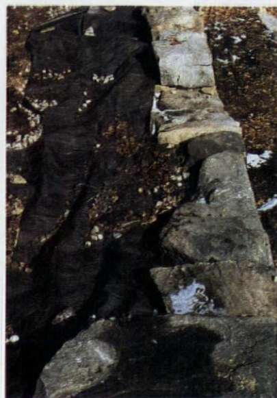
Landscaper's black filter paper is placed over the backing of a wall ready for topsoil.
