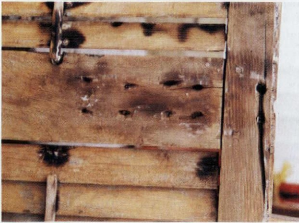
Stripped shutters revealed their problem spots. On this one, standard repair attempts of plugging screw holes with wood had failed and left bores, some as large as 1/2" in diameter.
