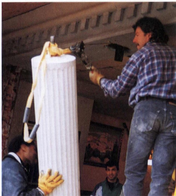
Once a column is finished, stainless-steel pins can be left in place to make handling and installation easier.
