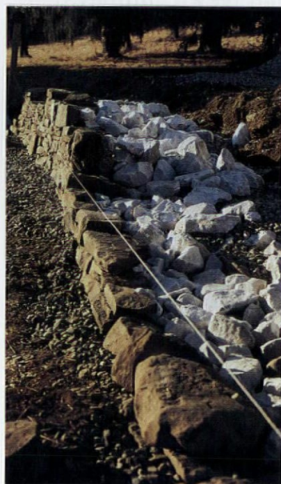
Since no one will see it, use cheap stone rather than nice fieldstone for backing. Here 5" to 8" limestone rip-rap came from a local quarry for $25 per ton.
