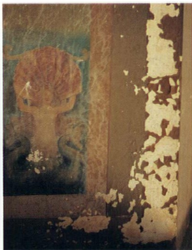
Severe moisture condensation has left runs and flaking on a century-old mural.
