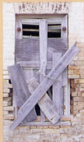
A common — but inappropriate — method of closing in that is as ineffective as it is unsightly.
