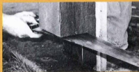
10" rotted bottoms of these load-bearing columns...
