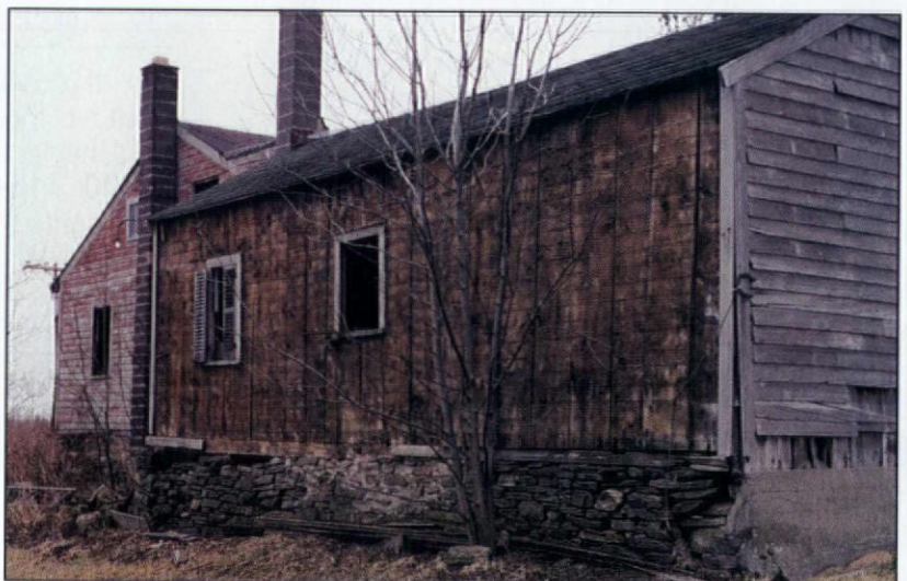
The vertical plank construction seen under the clapboards of this Ithaca, New York, house is a technique found across North America.
