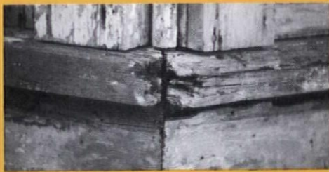
This rotted – and irreplaceable – woodwork...
