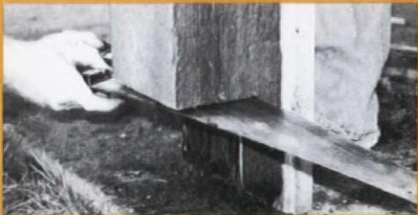
10" rotted bottoms of these load-bearing columns...
