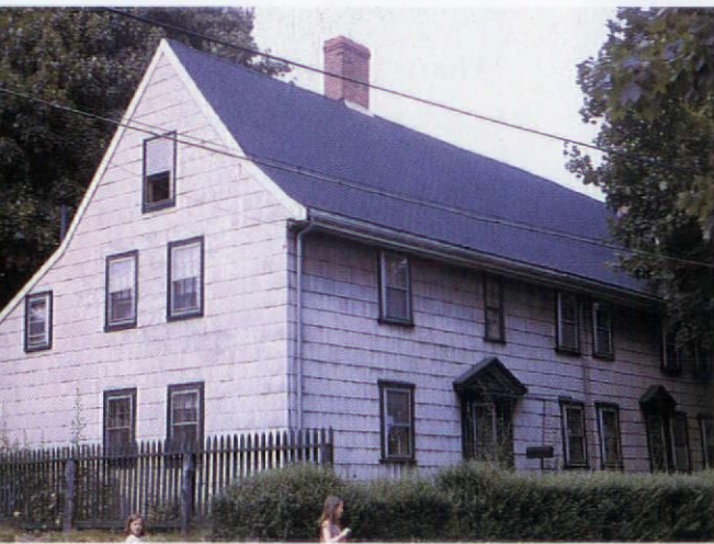
What's wrong with this picture? Could it be the 20th-century siding on the oldest house in Boston? (Pierce House, c. 1650)
