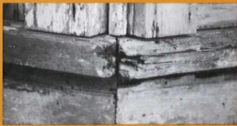
This rotted – and irreplaceable – woodwork...
