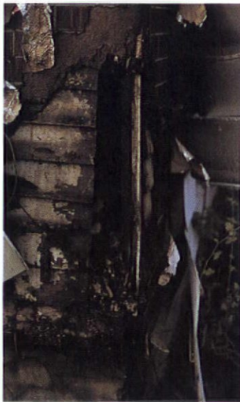
Three layers of material are peeled back to expose a hole that used to be the corner post.
