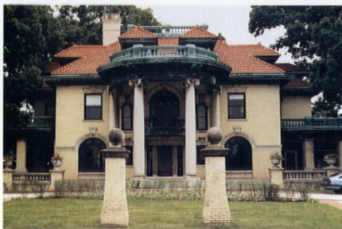
The stained copper balustrades and cornices of this Mediterranean-style mansion may respond to chemical cleaning or "agri-blasting."
