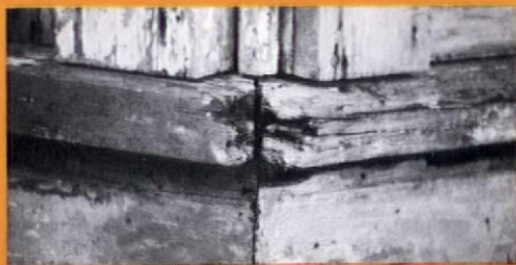
This rotted – and irreplaceable – woodwork...
