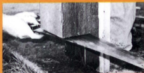
10" rotted bottoms of these load-bearing columns...
