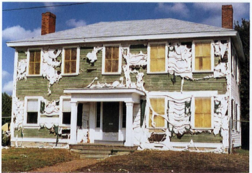
One removal method not covered in last issue's substitute siding article: Heat from a nearby fire melted this vinyl siding (and the shutters).
