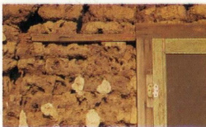
Individual sods and remnants of original clay-soil plaster show under the roof overhang. Like many sod houses that stayed in use, cement stucco was added in 1935.
