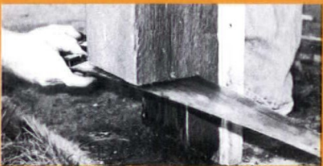
10" rotted bottoms of these load-bearing columns...
