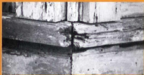
This rotted – and irreplaceable – woodwork...
