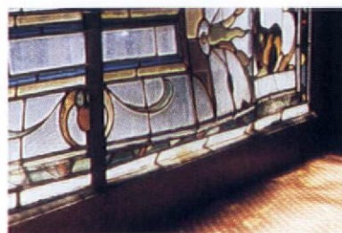
The weight of this window has defied the vertical reinforcing bars and caused a serious buckle.
