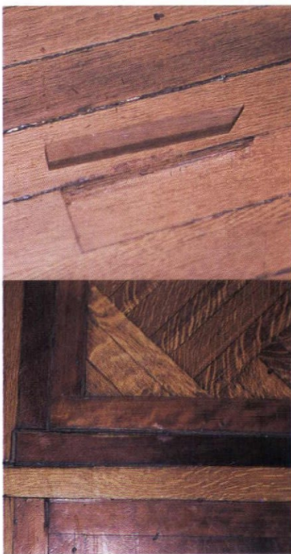
A dutchman repair using a patch of fireproof oak (cut first) to match the floor. Below: Typical broken shoulder damage—the price of oversanding.
