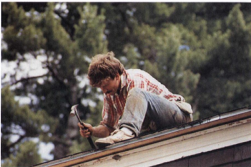
Loose shingles, ice dams, and holes punched by branches kept us busy on the roof more than once over the years. Here Curt is working on the first reshingling project.
