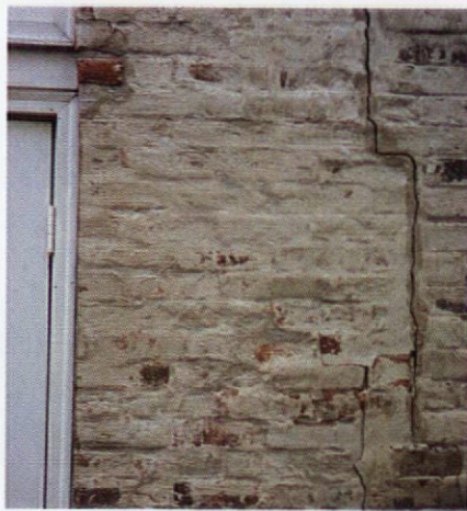
Chipped brick, sloppy repairs, and goeey overcoats can mean repointing is not enough to resurrect the wall.
