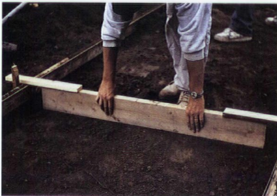
As it is pulled along the forms, the 6" screed board levels the earth, which is now ready for a layer of stone dust.
