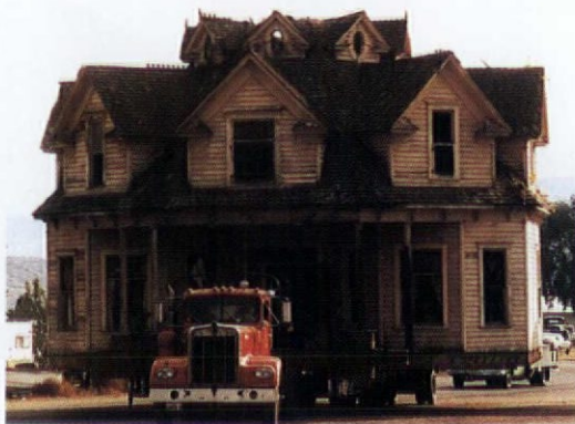
Relocating Cecile Allen's octagon house required removing its steeple-like roof tip in order to clear power lines.
