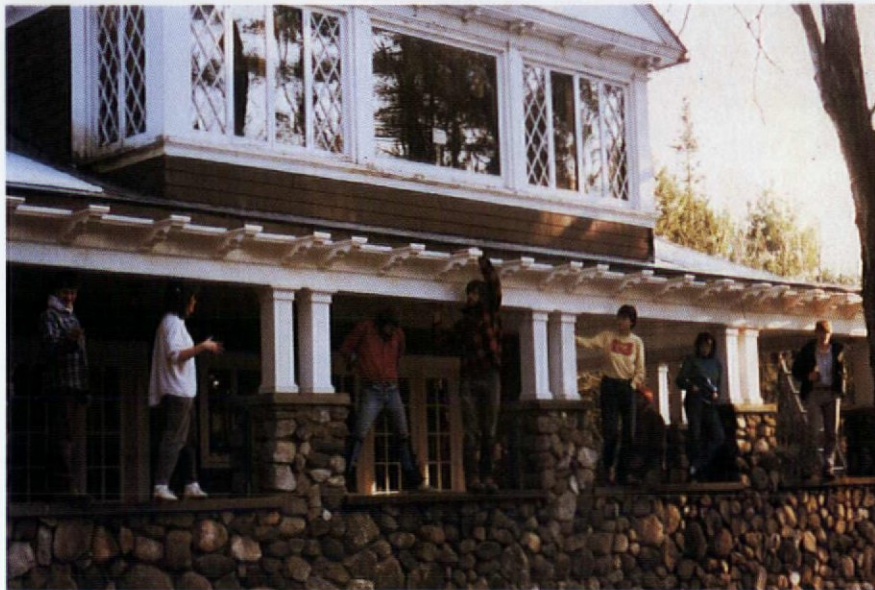
Little did we know when this photo was taken that the support beams below the second-floor master bedroom were rotting.
