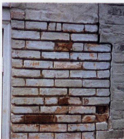
Resurfacing involves clearing mortar joints as if repointing, and then filling voids in brick.
