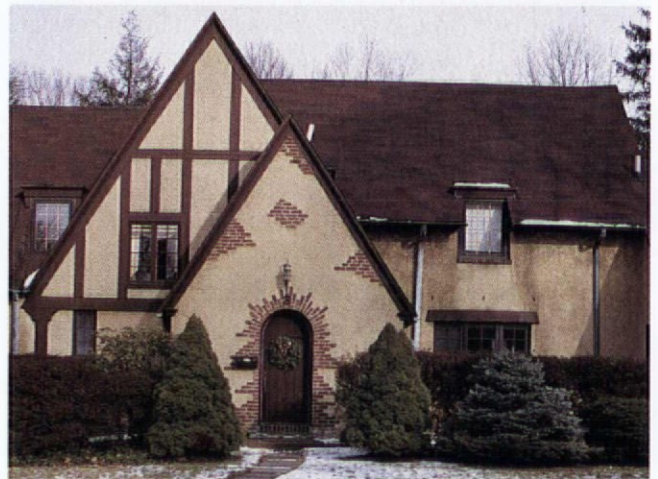
A Tudor in Wallingford, Pennsylvania with classic use of brick patches peeking through the facade stucco.
