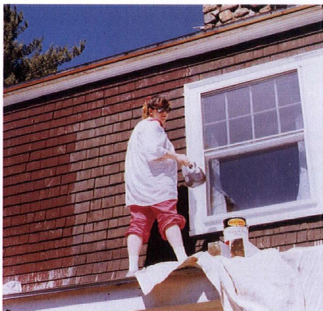
A coating of chocolate brown paint with white trim gives the place a "gingerbread house" appearance. The paint job was one of the many home improvement projects Karin (above) and I tackled in the summer of 1990.
