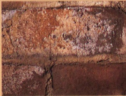
Efflorescence — a sign of moisture.
