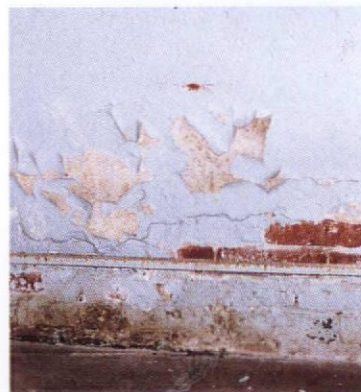
Peeling paint and plaster, along with musty smells, are classic symptoms of rising damp.
