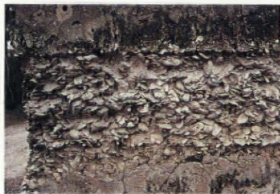
One course of tabby on this 1820s house in Sapelo Island, Georgia, has lost its parging, exposing the oyster-shell aggregate.
