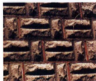
ABOVE: Surprising details enliven the regularity of many block buildings: belt course of delicate cast copings (top); woven-wall pattern produced by a "triple stone" design mold. INSET: Concrete block turned to the Colonial Revival in upstate New York.
