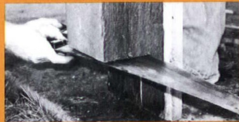
10" rotted bottoms of these load-bearing columns...
