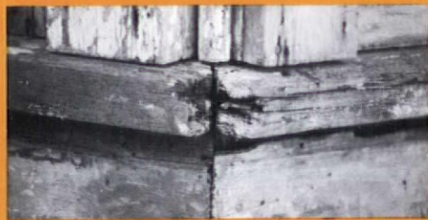
This rotted – and irreplaceable – woodwork...
