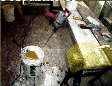
MIX finish lime and pigment in a 5-gallon bucket using a drill with blade attachment.
