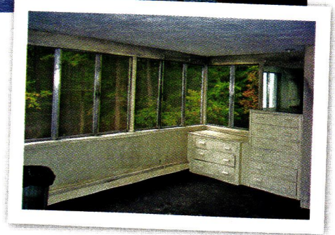
The window frames upstairs weren't damaged in the fire, but were fitted with new double-paned glass for energy efficiency.
