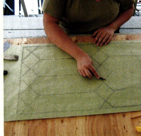
ABOVE: Create a template—a roadmap to repairs—by tracing the window on paper.
