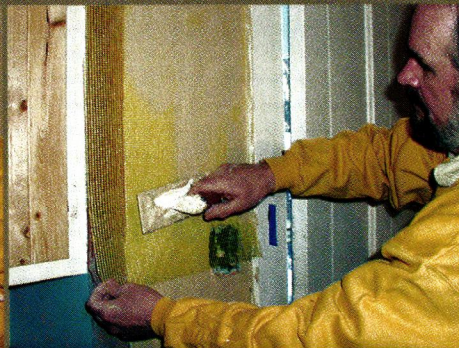
LAYER nylon mesh over cracks, embedding it into the first coat of plaster.
