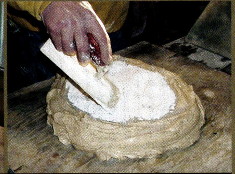
ADD gauging plaster to the water, and mix it all together with a short trowel.
