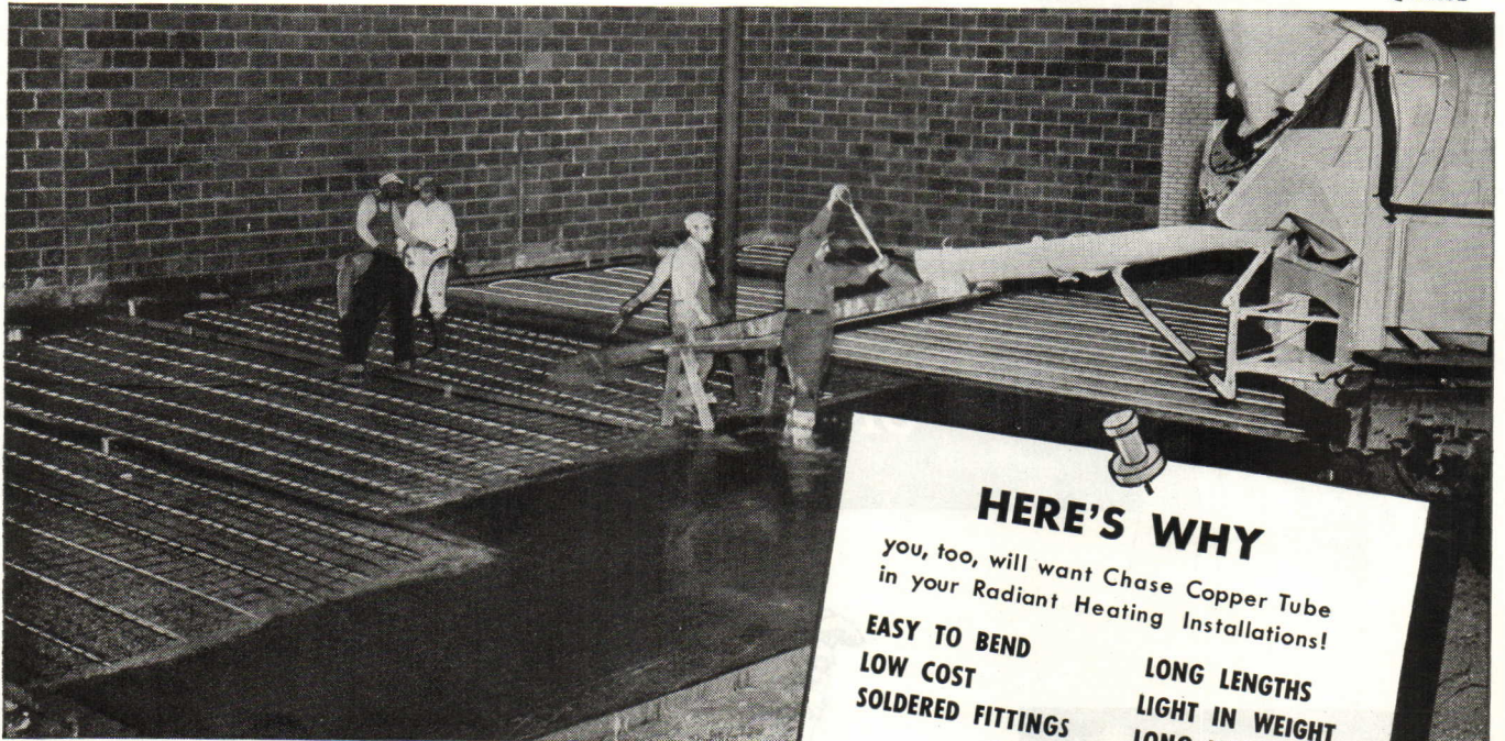
Pouring concrete over 12,000 feet of Chase Copper Tube. Installation also included 5500 feet for office ceiling and 1200 feet for sidewalk and drive snow removal. Architect: Charles A. Maguire & Associates, Providence, R. I. Building Contractor: A. F. Smiley Construction Co., Pawtucket, R. I. Heating Contractor: J. F. Higgins Heating Co., Providence, R. I.
