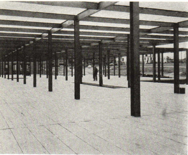
Fenestra's "Holorib" decking (Detroit Steel Products Co.) used on the Mechanical Bldg., Adelphian Academy, Holly, Mich.; Charles W. Nicol, architect.
