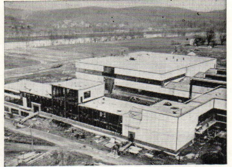
42,000 square feet of Cemesto used for roof deck and curtain walls. B. F. Goodrich Co., Marietta, O.
