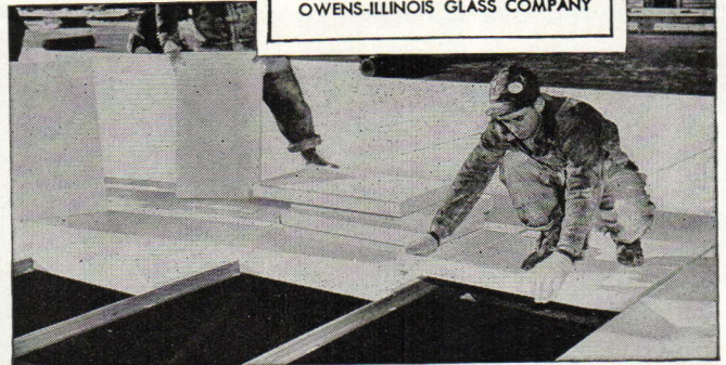
Ease of handling is seen here, as lightweight Kaylo Roof Tile is slipped into place on sub-purlins.
