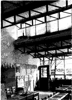
Figure 2—view of end-on classroom facing east-southeast. Although subsequent tests proved them unnecessary, steam mains were installed below clerestory windows to overcome anticipated cold “down draft.”
