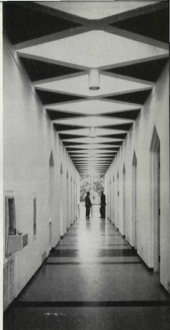
X-SHAPED BEAMS create diamond-shaped skylights in the central corridor where precast roof segments meet.
