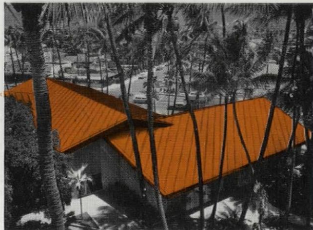
MOST UNUSUAL ROOF EFFECT is obtained by running batten seams on the diagonal. Copper was furnished by Revere Copper and Brass Incorporated. Architect: VLADIMIR OSSIFOFF, F.A.I.A.
