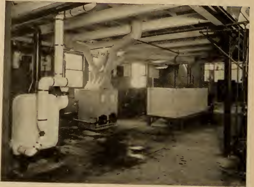
HEATING EQUIPMENT IN ACTUAL OPERATION, SHOWING HOW IT IS INSTALLED IN THE LABORATORY
