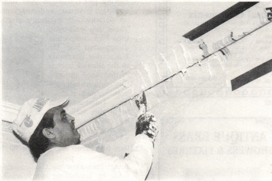
Peel-Away I is applied like joint compound to a depth of about 1/4 in. on the surface to be stripped. A test patch establishes optimum thickness and soak time.
