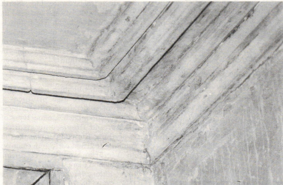
After soaking for 24 hr., the blanket is stripped off, peeling the paint with it. Disposal of paint-laden blanket should comply with regulations for lead materials.
