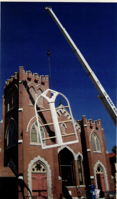
Bovard Studio built and installed a replacement frame for the stained-glass window for Immanuel Lutheran Church in Pensacola, FL.
