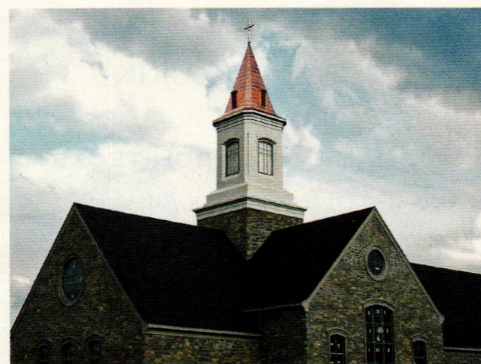
This prefabricated steeple with a copper spire and cross was fabricated by Munns Manufacturing for the Horizon Community Church in Cincinnati, OH.
