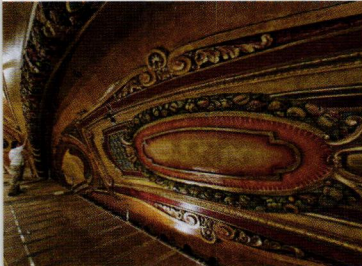
Restoration of the ceiling at the Buffalo Performing Arts, an historic movie palace in Buffalo, NY, in 1926, now hosts traveling Broadway shows, thanks to a renovation by Swiatek Studios .
