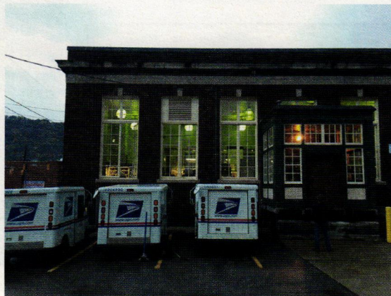
Allegheny Restoration restored these windows for the post office in Monongahela, PA. Click on no. 1004
