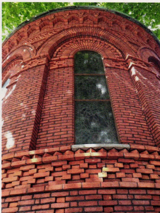
LimeWorks.us provides restoration and repointing services for masonry projects. Click on no. 2083.
