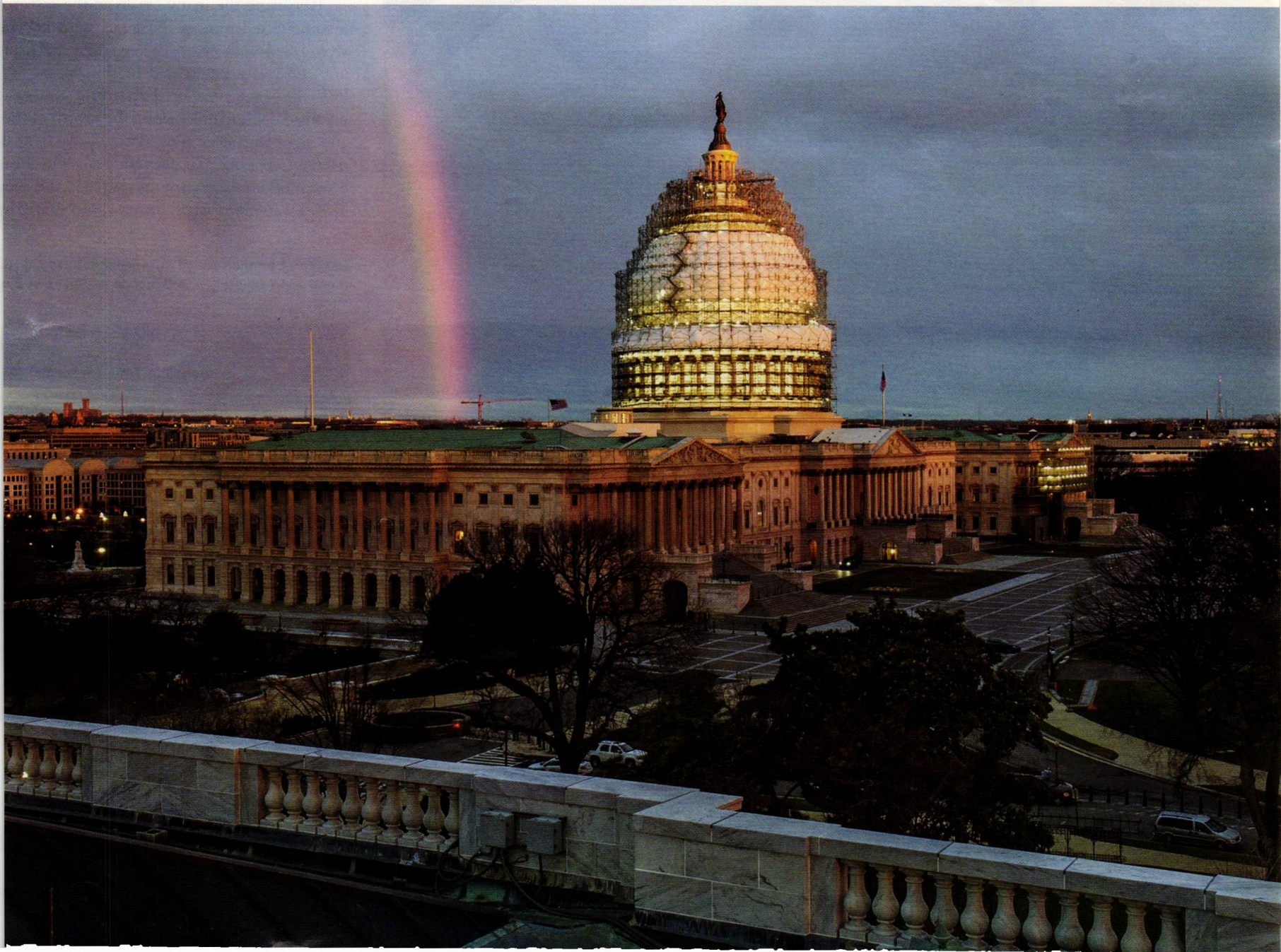
RIGHT & BELOW: Scaffolding on the exterior included 52 miles of scaffold piping on 25 levels, and two miles of decking.
