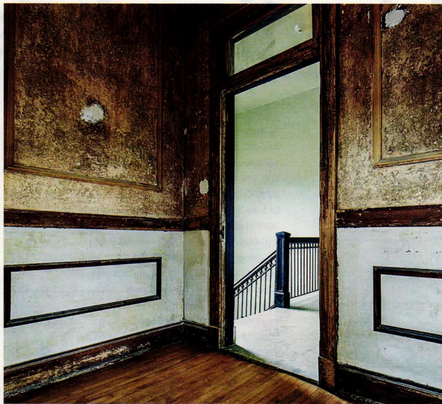
LEFT: A reclaimed office space on the third floor illustrates the team's "leave-alone" principle. Photo: Photo: Steve Hall © Hedrich Blessing
