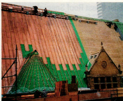
Heather & Little's restoration of the Toronto Old City Hall required 113,900 sq.ft. of copper roofing, cornices, gutters and sheet-lead work.
