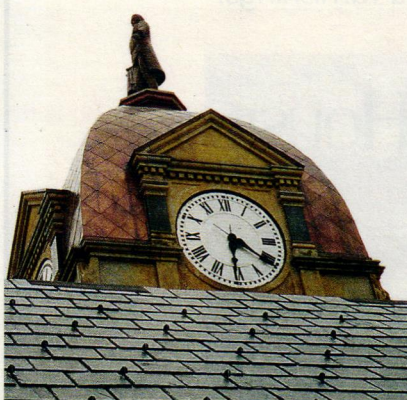
NIKO replaced the slate roof and sheathed the clock-tower dome in copper on the Hancock County Courthouse in Findlay, OH.
