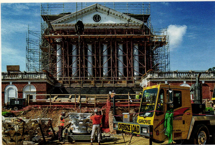
LEFT: Temporary steel shoring was erected to support the portico roof structure during the removal and replacement of the marble column capitals. The copper sheet metal cornice installed by Stanford White following the disastrous 1895 fire, was removed, stripped of paint, refinished and reinstalled on restored cast-iron framing brackets. The existing north marble stair was dismantled, cleaned, repaired and re-installed above a new waterproof membrane protecting the building construction below.
