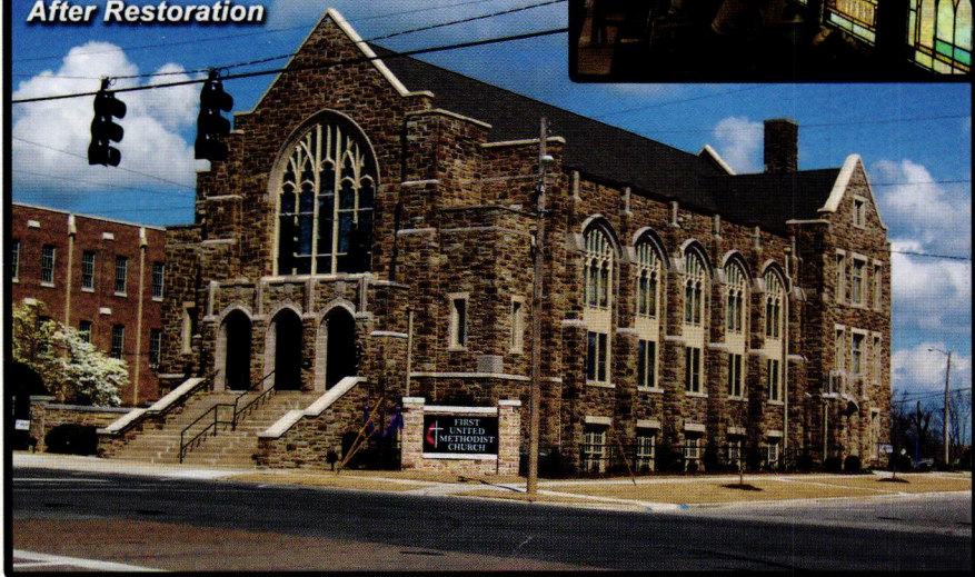
Before and after photos of the F4 tornado damage to the First United Methodist Church of Cullman, Alabama restored by Bovard Studio Inc
