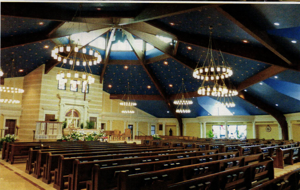
At Saint Elizabeth Ann Seton Parish in Pickerington, OH, the interior, including its ceilings and flooring, was gutted, leaving the structural wood-lam framing as a starting point.
