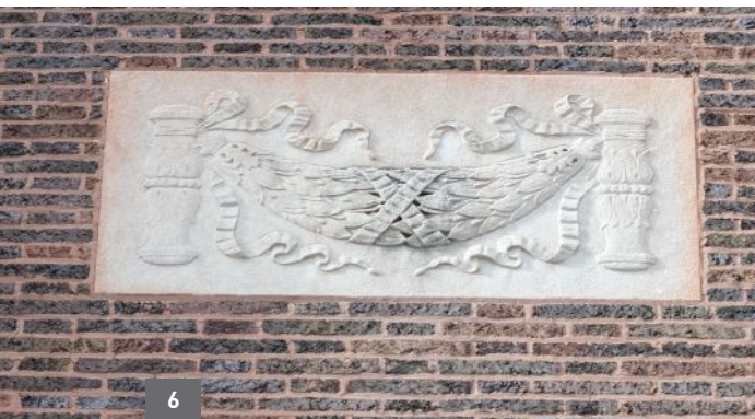
6 Unstable colorant was used in the mortar, resulting in staining of the stone work.
