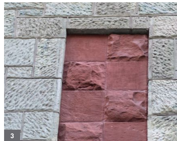
4 Deteriorated fine mortar joints showing cracked, separating, eroded and missing mortar.
