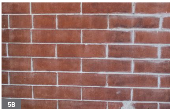
5B A narrow mortar joint was partially repointed, using too thick of a saw cut, resulting in widening of the joint.
