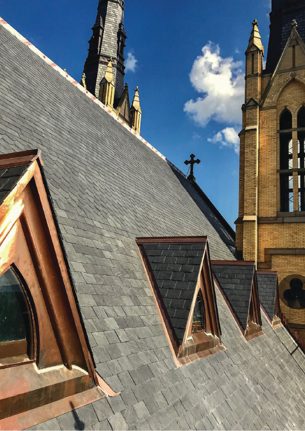
ABOVE Critical to the integrity and beauty of the new roof is new copperwork in valleys, ridges, and dormer and spire details.
