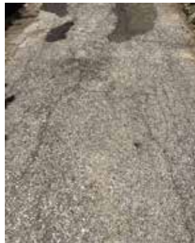
Cracking in driveway
