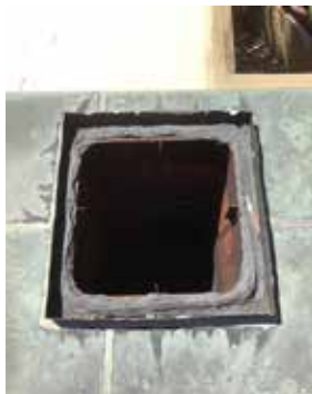
Rain screen and cap needed
