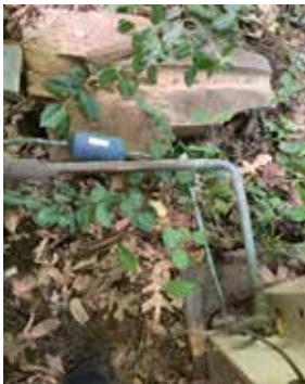
Refrigerant line housing is missing
