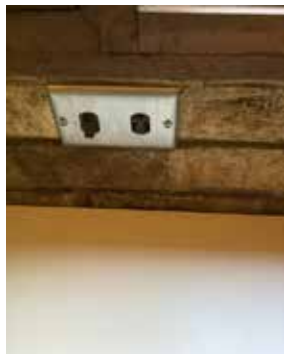
Outlet near kitchen sink should be GFCI
