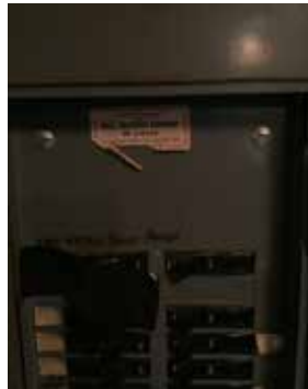
No main switch
