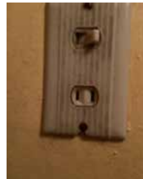
Two prong outlets
