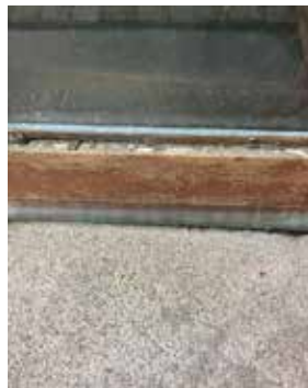
Missing window trim
