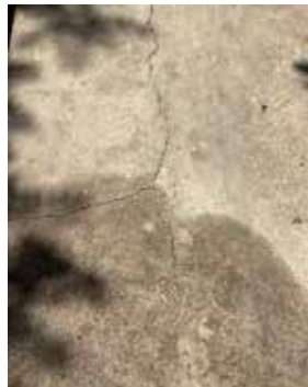
Cracking in front patio
