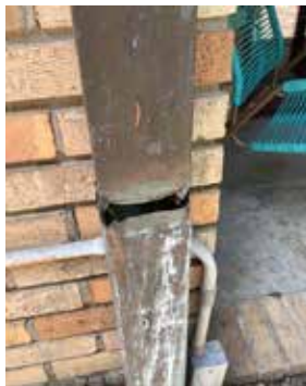
Separation in downspout
