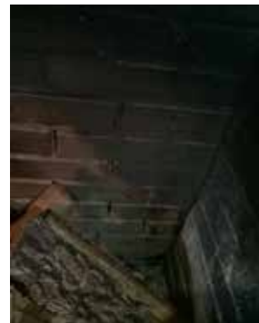
Gaps in grout
