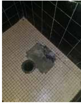
Damaged floor tile
