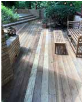
Deck needs paint/stain
