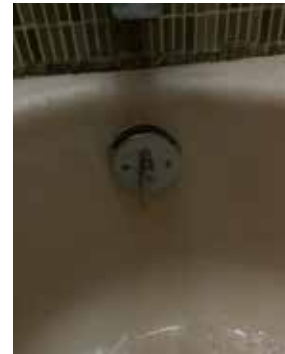
Inoperative drain lever
