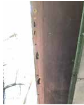
Carpenter bee damage
