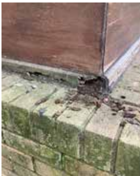
Wood rot on the rear of the home
