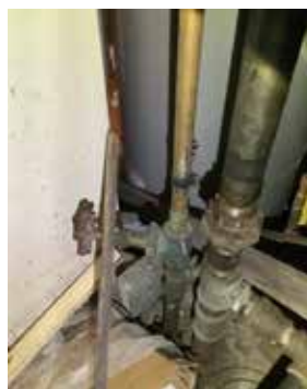
Near water heater
