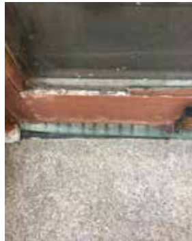
Damaged window trim
