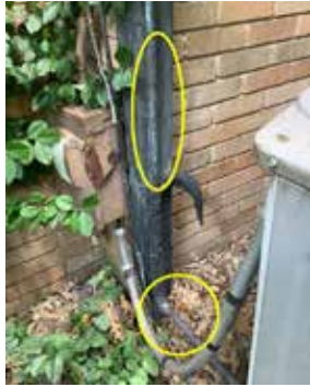
Refrigerant line housing is missing
