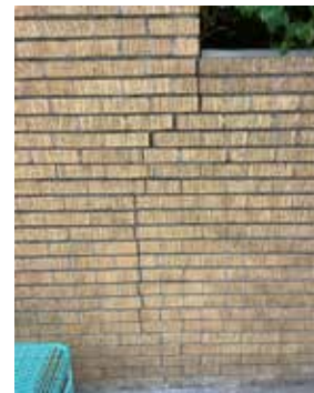
Cracking in retaining wall
