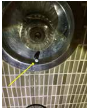
Inoperative diverter valve
