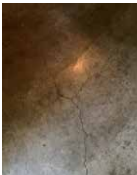
Cracks in floor
