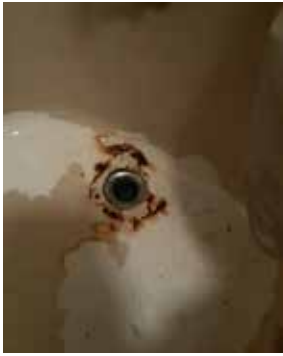
Rust in bath tub
