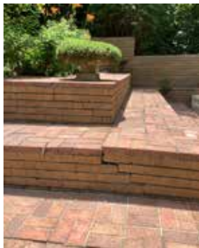
Cracking in brick retaining wall
