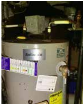
Reliance 40 gallon, gas unit
