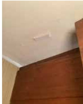
Peeling plaster in bathroom ceiling
