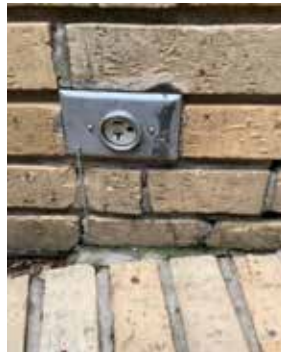
Outlet missing cover
