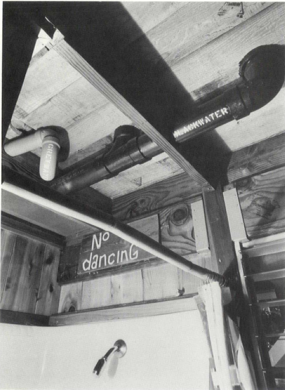
Plumbing is exposed and readily accessible.
