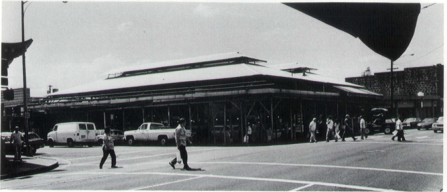
It was business as usual during Phase I construction on Oahu Market. New owners received grants to fund the rehabilitation project. Photo by Phil Haisley.
