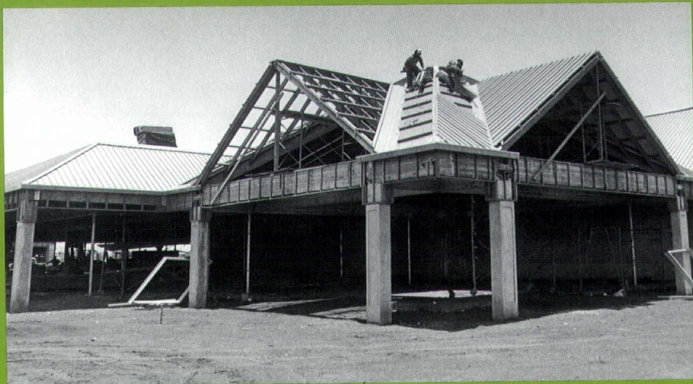
Construction workers apply blue Dimondek® metal sheeting to the roof of the future Mililani Town Center. The shopping center, with planned additional phases, will be the largest in Hawaii. Photo by Jamie Kemp
