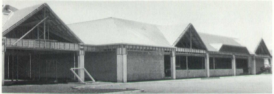
Roofing is in place at certain areas of the shopping center, which is scheduled to open late this year.
