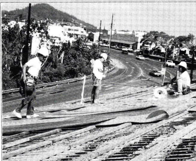
Kauai Civic Center After Hurricane Iniki
