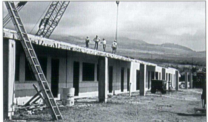
The work diligently continues on the classroom building of the new Kihei school.
