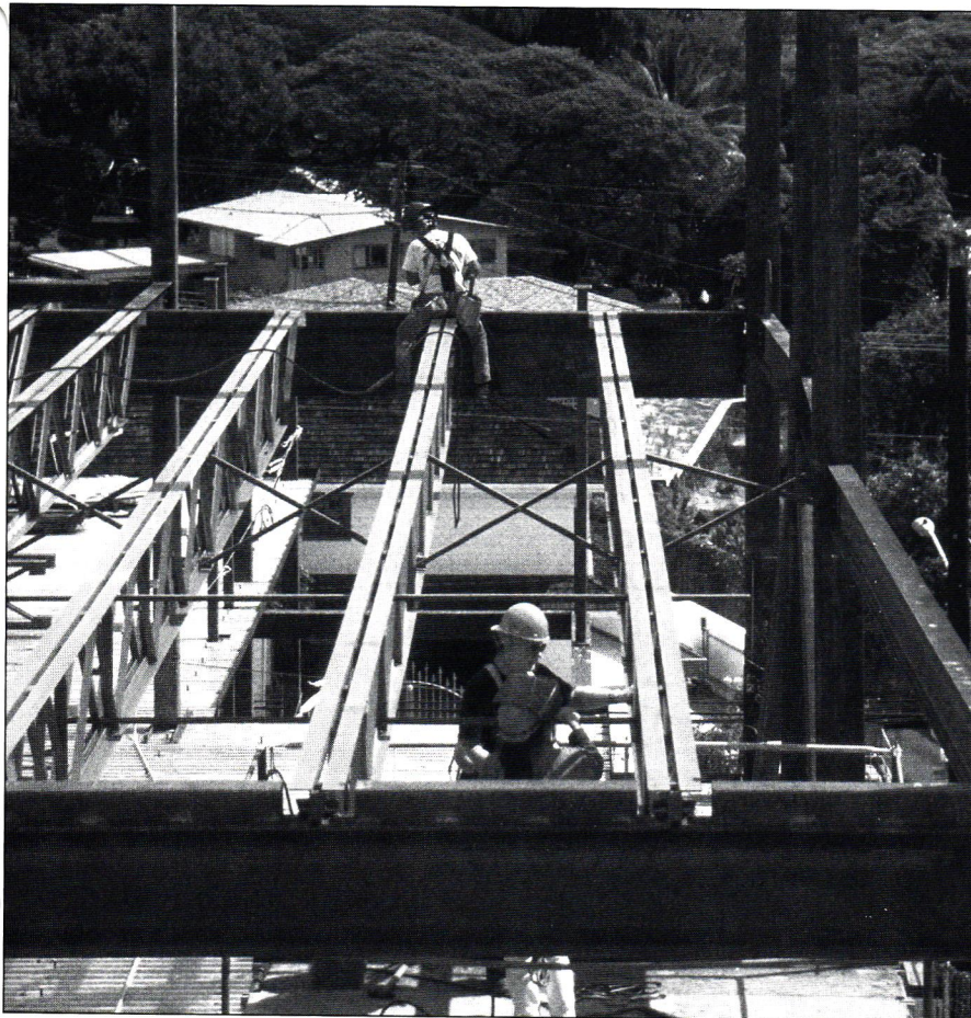
Shown here is the 47-foot span open web joist at the second floor.
